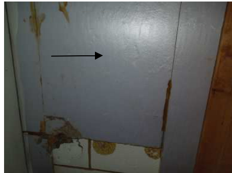
Unprotected foam insulation in basement
