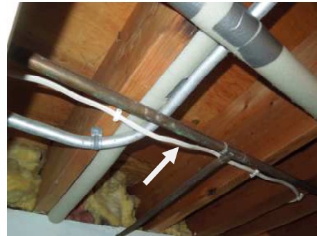
Unprotected romex type wiring in basement
