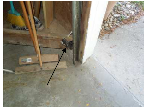
Electric eyes at overhead door higher than recommended
