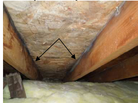
Dark staining at roof framing
