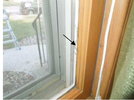
Cracking at glass in living room window
