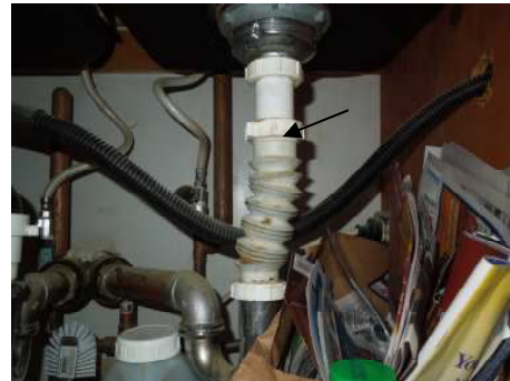
Flexible drain piping under various sinks
