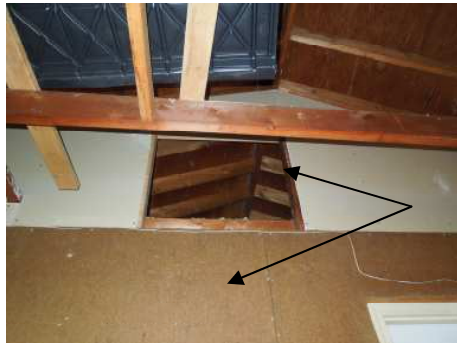
Firewall not installed between house and garage
