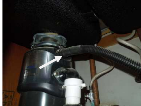
Air gap not installed at dishwasher drain
