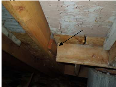
Loose framing around chimney in attic
