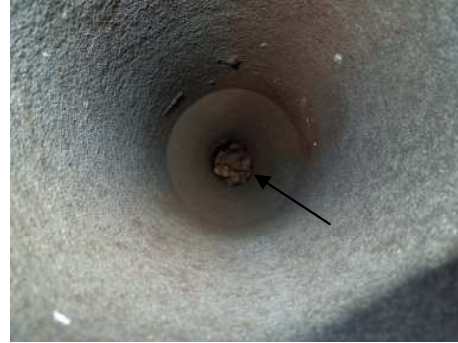
Plumbing vent partially obstructed
