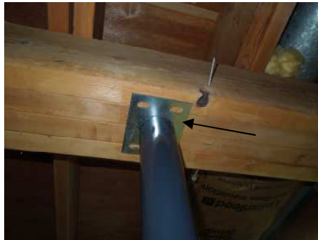
Support column not permanently secured
