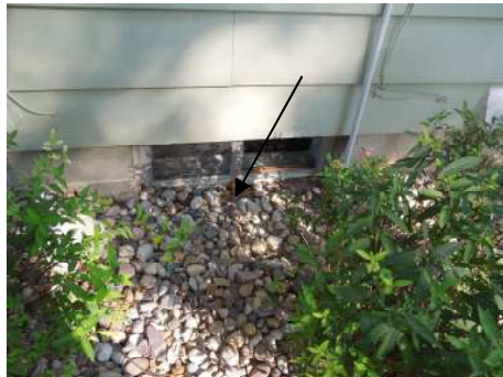
Recommend window wells and covers at basement windows
