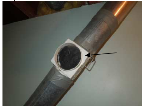
Recommend removing device at dryer vent
