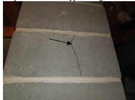
Recommend sealing crack in chimney in basement
