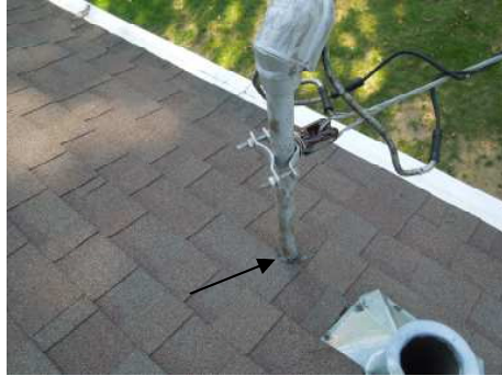
Flashing not installed at electrical conduit
